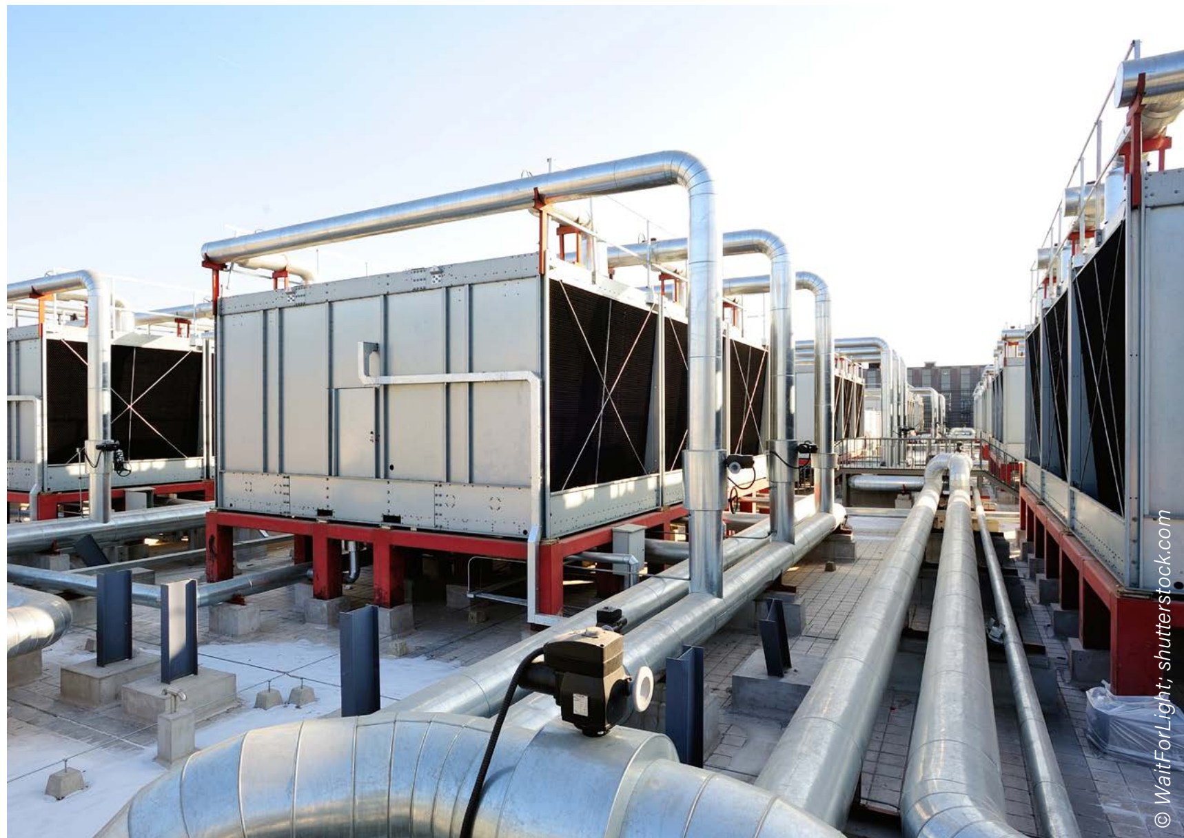
Sets of cooling towers in the data center
