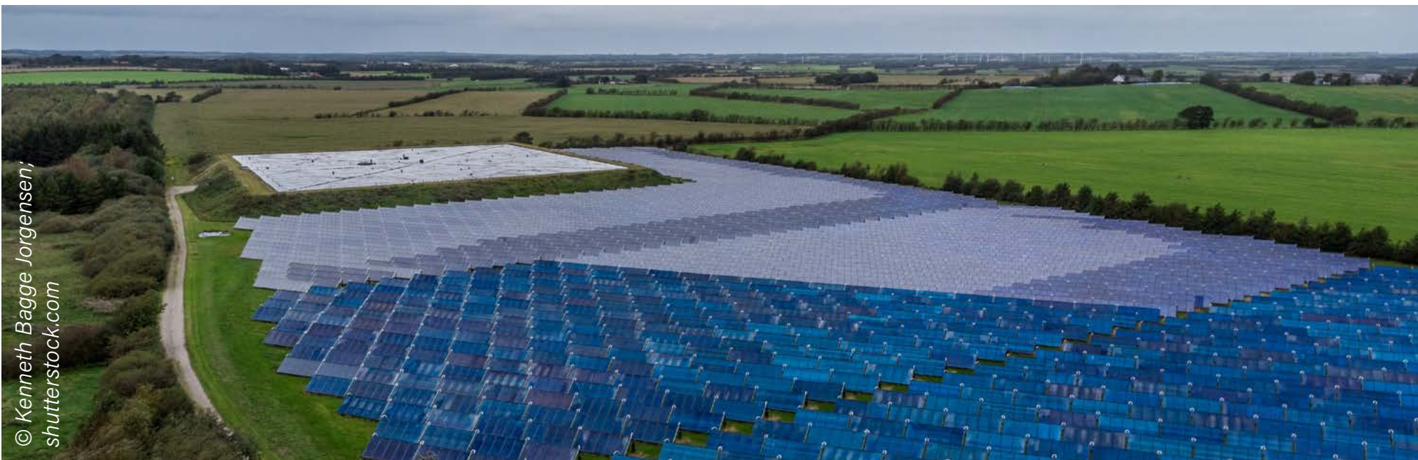
Toftlund District Heating Solar Park, Denmark
