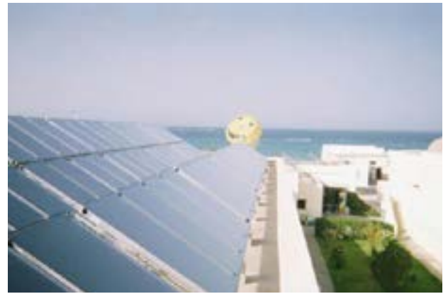
SWH on hotel rooftop in Tunisia, Prosol Tertiary SWH programme
