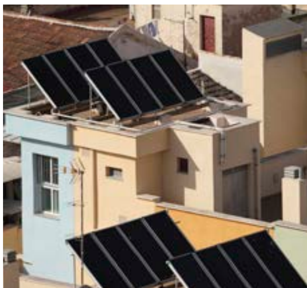
Solar water heating systems on residential rooftops
